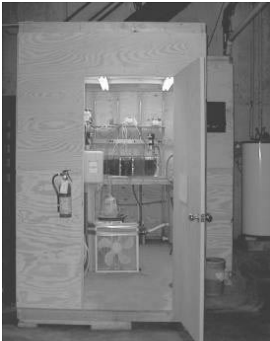
Figure3a - Reactor building constructed to maintain reasonable operating temperatures.
